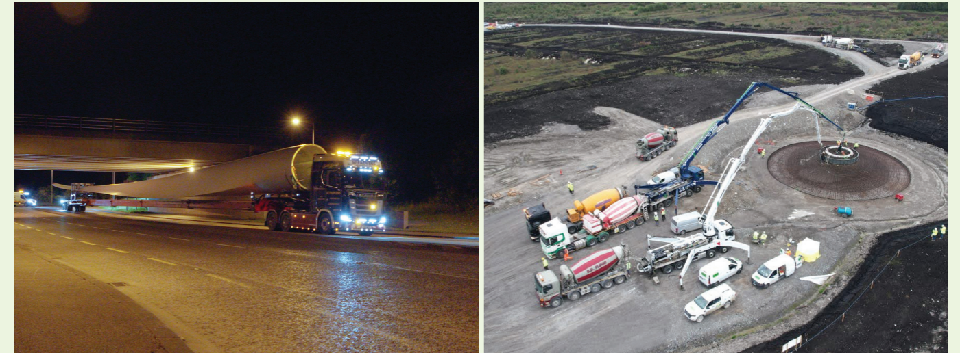
Figure 4 The delivery of wind turbines to site. Figure 5 Preparing for the concrete pour for the first turbine's foundation.
